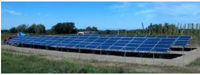
The Cornell Lake Erie Research and Extension Lab's solar arrays generate about 30% of the electrical energy used by the Lab.
