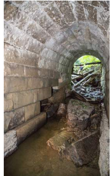
This eroding culvert poses a threat not only to stream quality, but to the Rail-to-Trail which passes over it. Photo Credit: Chautauqua Rails to Trails.
